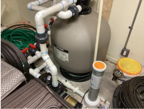
Pool mechanical equipment
