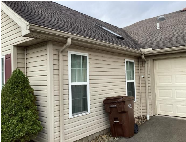
Aluminum gutters and downspouts
