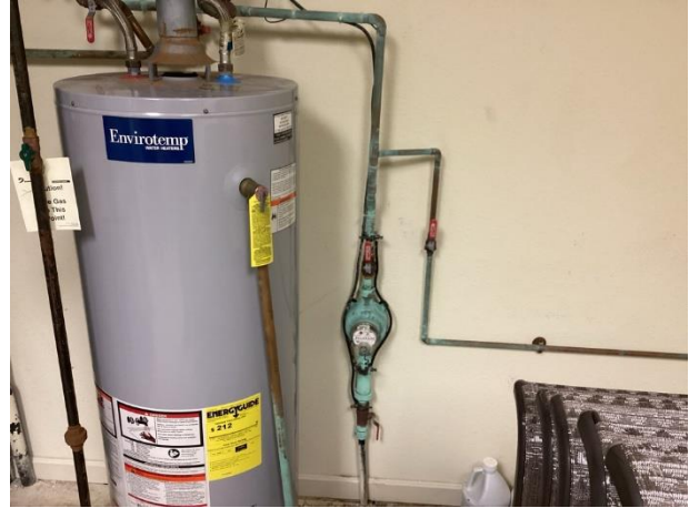
Corroded copper piping
