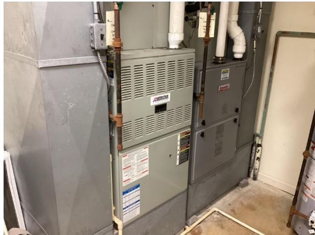
Split system air handling unit
