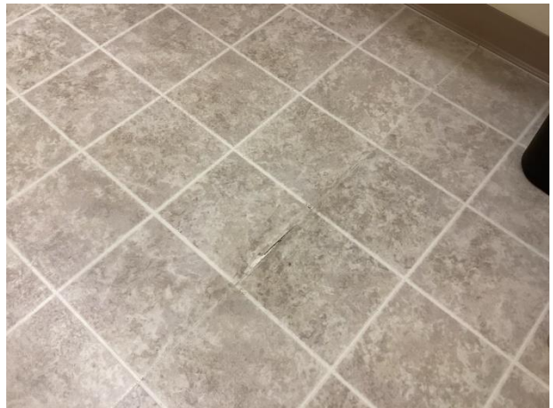
Damage to the vinyl floor coverings
