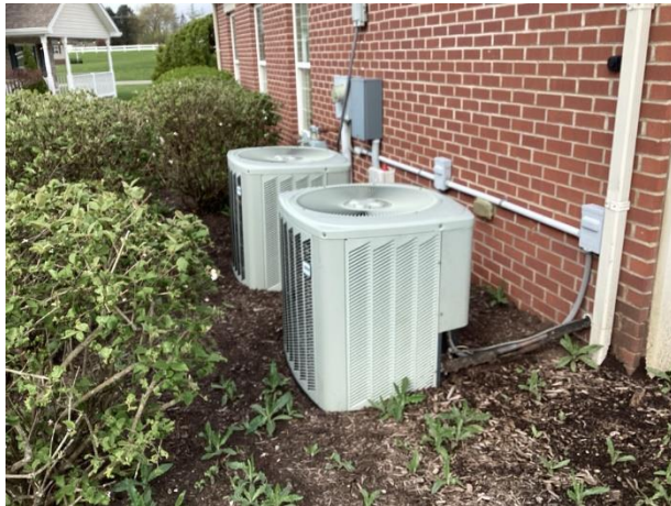
Split system condensing units
