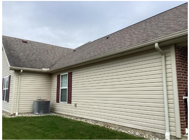
Aluminum gutters and downspouts
